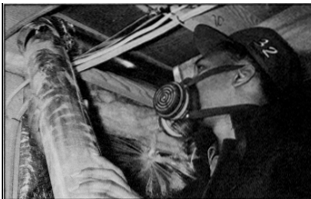
Heating and air conditioning ducts can accumulate dust that contains lead.
